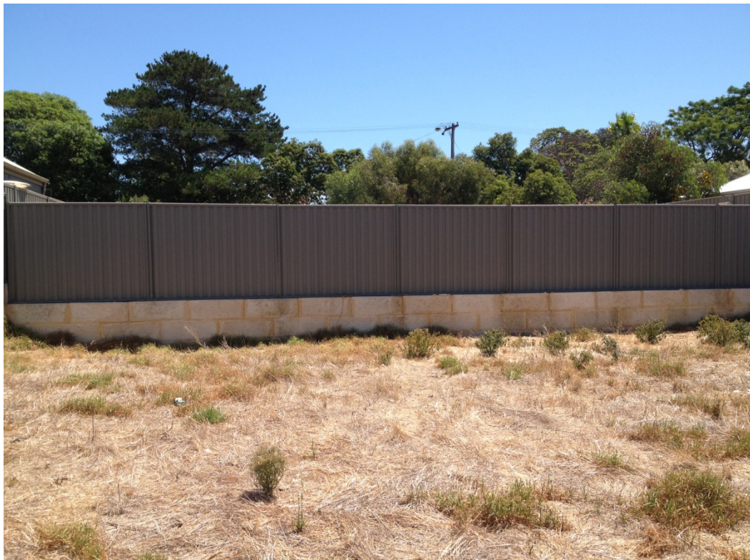
Existing retaining wall adjoining No. 46 Hines Road, Hilton as viewed from the land.
