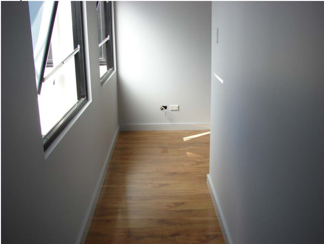
Photograph 2 – passageway at first floor level – northern side – refer to Item No. F2
