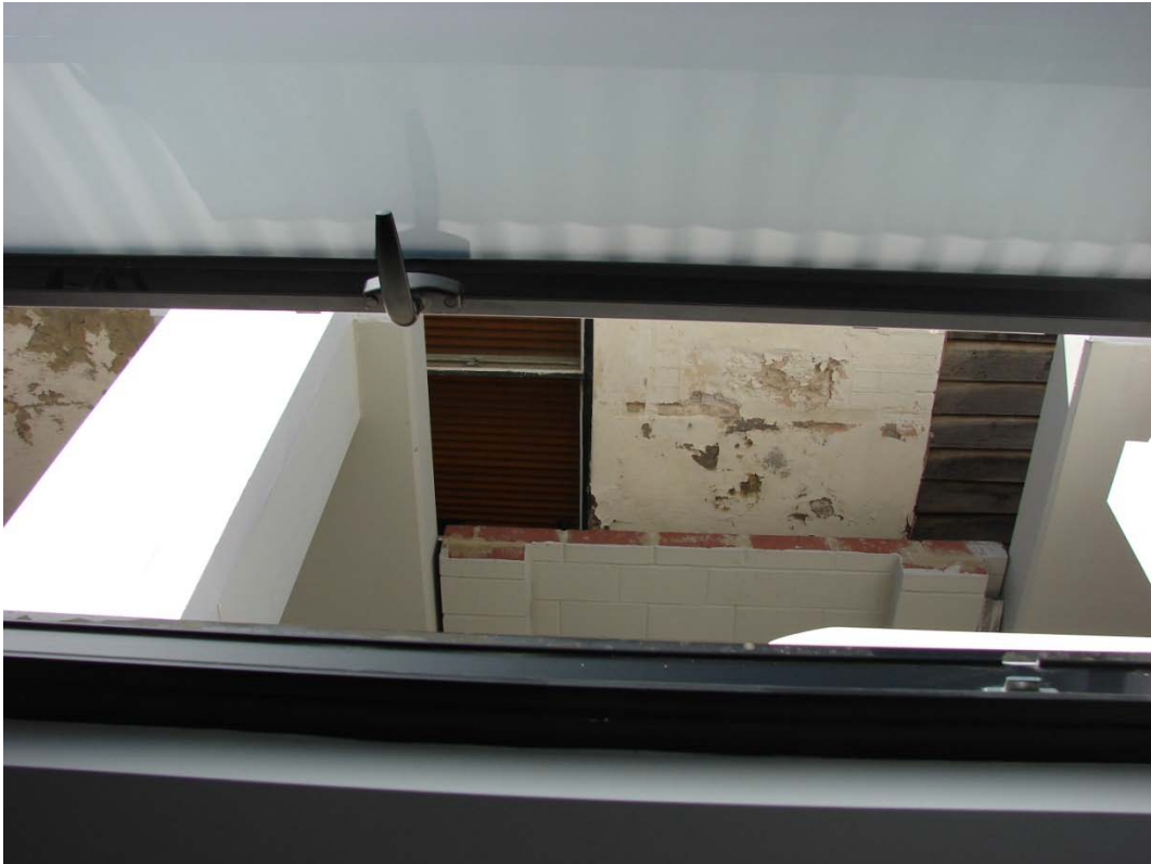
Photograph 3 – taken in passageway looking towards 86 Marine terrace – refer to Item No. F2 of report
