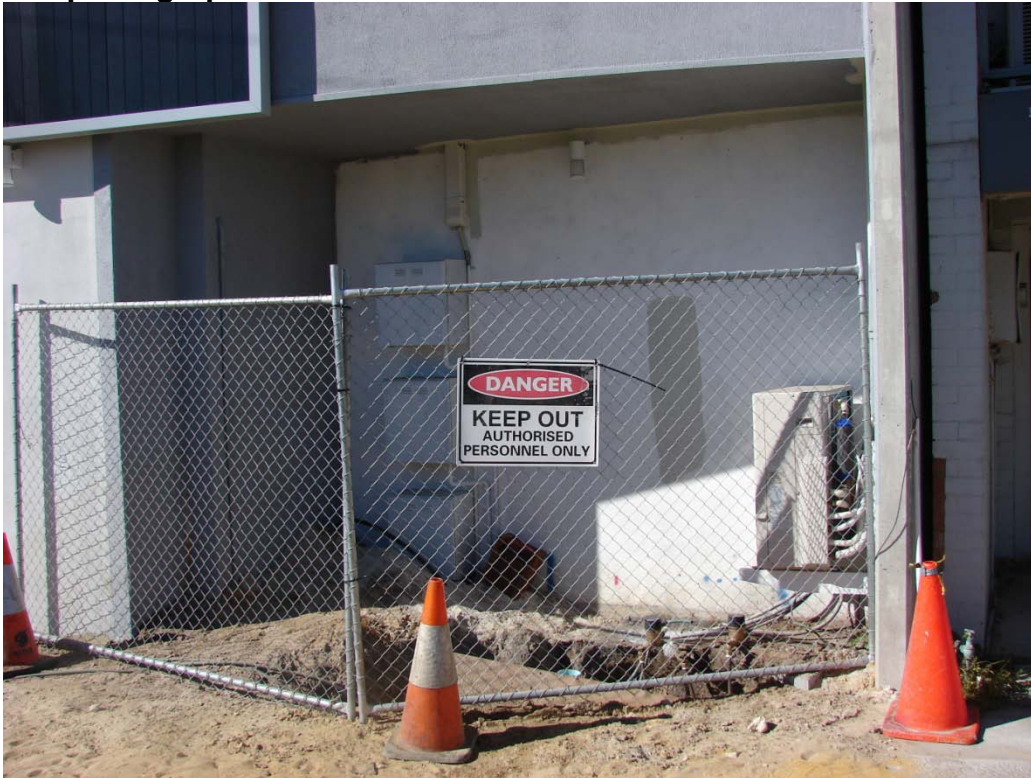
Photograph 1 – unauthorised service area to Marine Terrace – Refer to Item No. G1 of report.
