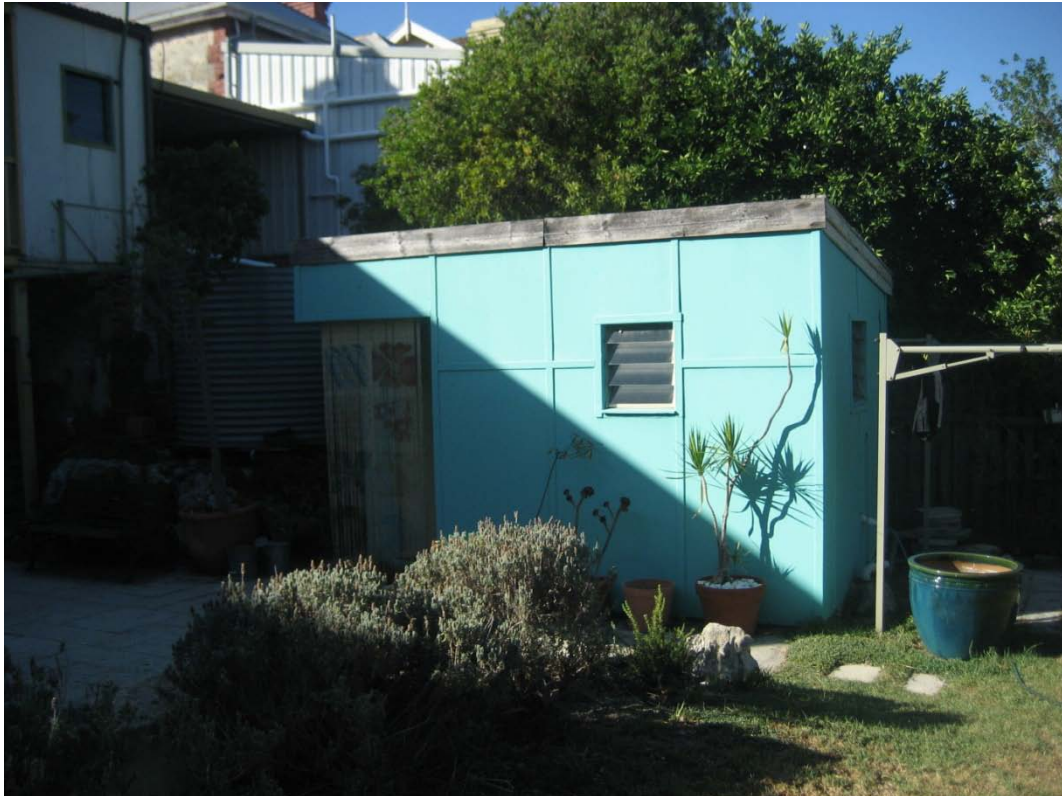
View of the existing Storeroom at the rear of the land to be retained and re-cladded.
