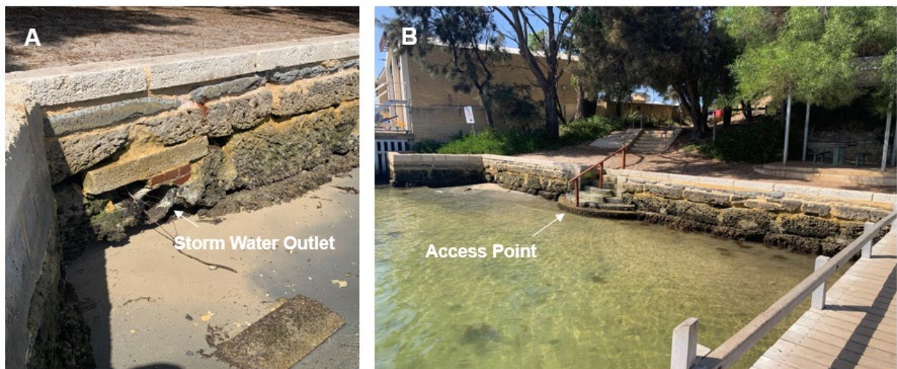
Figure 3-3: Storm water outlet (A), Southern Harvey beach shoreline and the steps used for entry into the water and one of two picnic tables (B).
