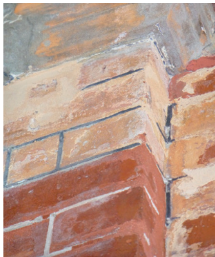
Remnants of 1890s tuck-pointing of bichrome brickwork.
