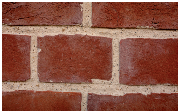
Damage to brickwork from the use of an angle grinder or disc cutter. The torque produced by rotating tools makes them difficult to control. (Photograph: David Young)
