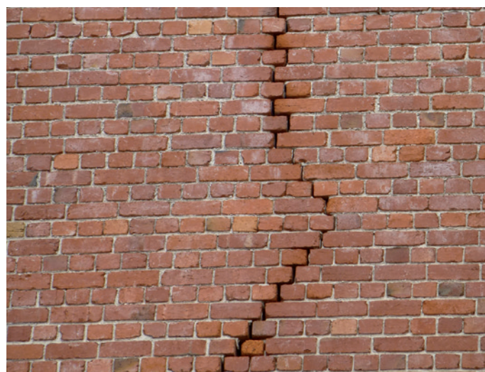
Always get a Structural Engineer to check cracks in case remedial works need to be carried out.
