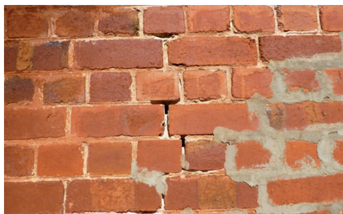
This wall requires repointing to replace deteriorated mortar joints as well as poor maintenance work from the past which has used damaging cement mortar.
