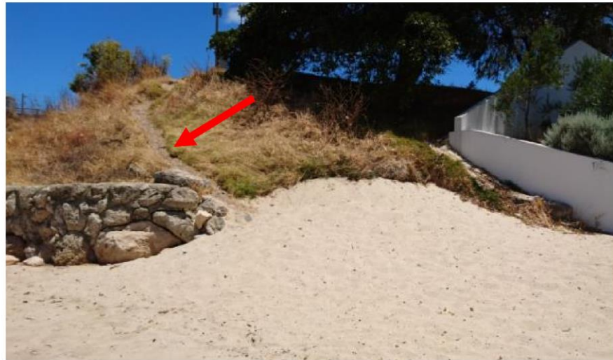
Figure 2-11 Exposed foot trail on traffic bridge abutment and carpark embankment.
