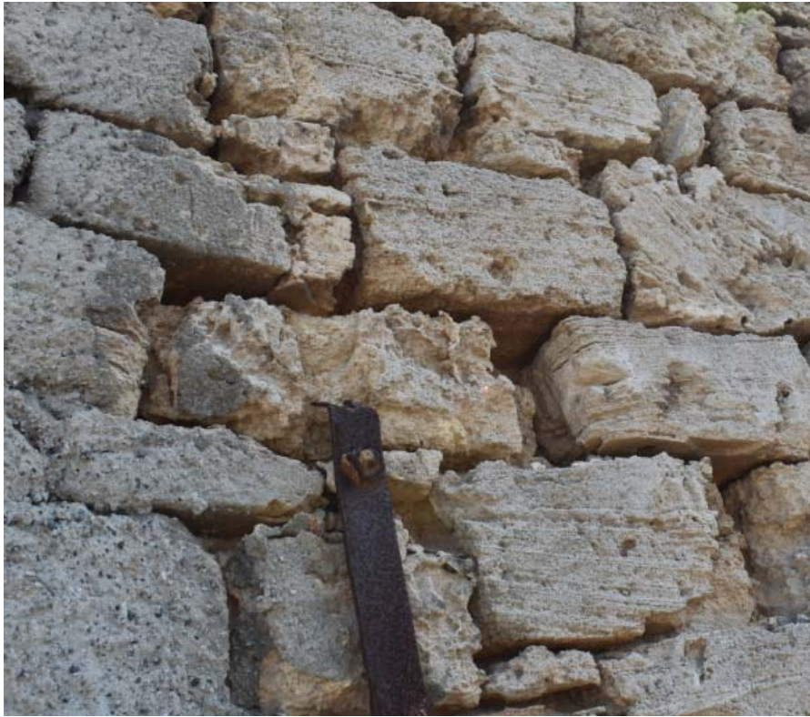
Next to this masonry wall is an area where shotcrete has been applied in an apparent attempt to prevent the erosion and fretting of the upper part of the cliff within the 'zone of roots.' The shotcrete does not appear to have adhered well to the sandy friable surface of the limestone and cracks can be seen (see photo below). Pieces of shotcrete now present a rockfall hazard.
