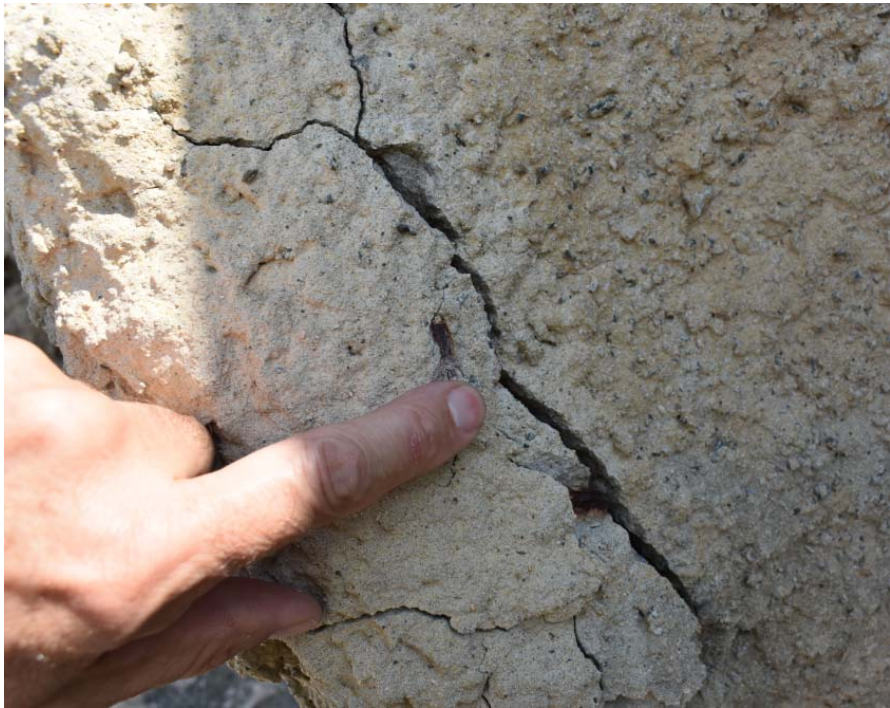
Further west the 'zone of roots' section of the face is particularly friable and it is from this section that a large pinnacle of material (approx. 100 kg)
