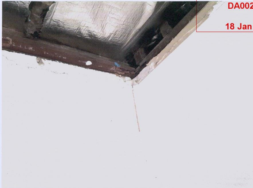
WHITE ANT DAMAGE INTERNAL
