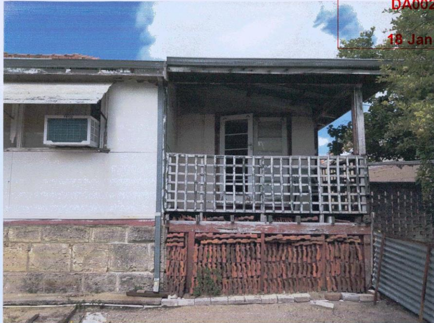
SLIPPAGE, SW CORNER
