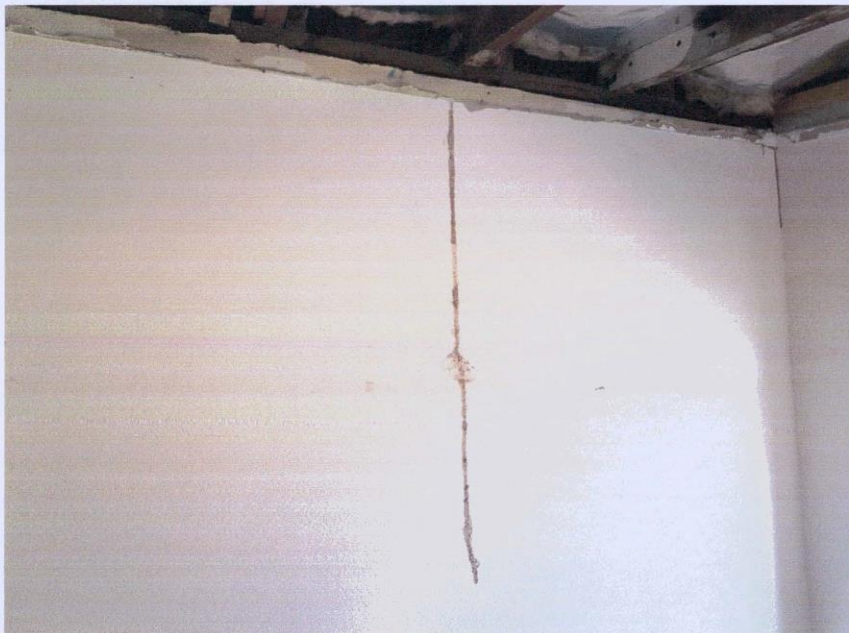
WHITE ANT DAMAGE INTERNAL
