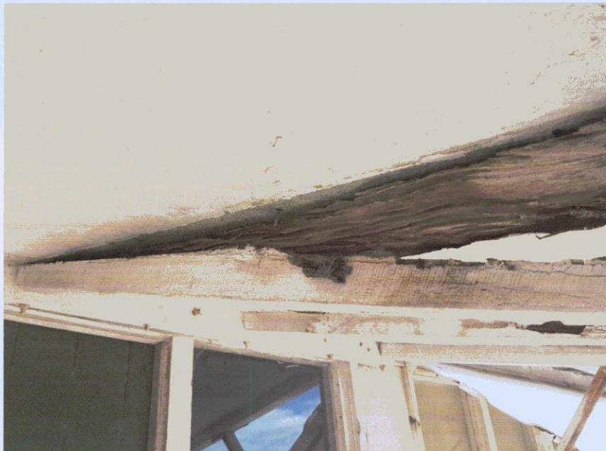
WHITE ANT DAMAGE EXTERNAL
