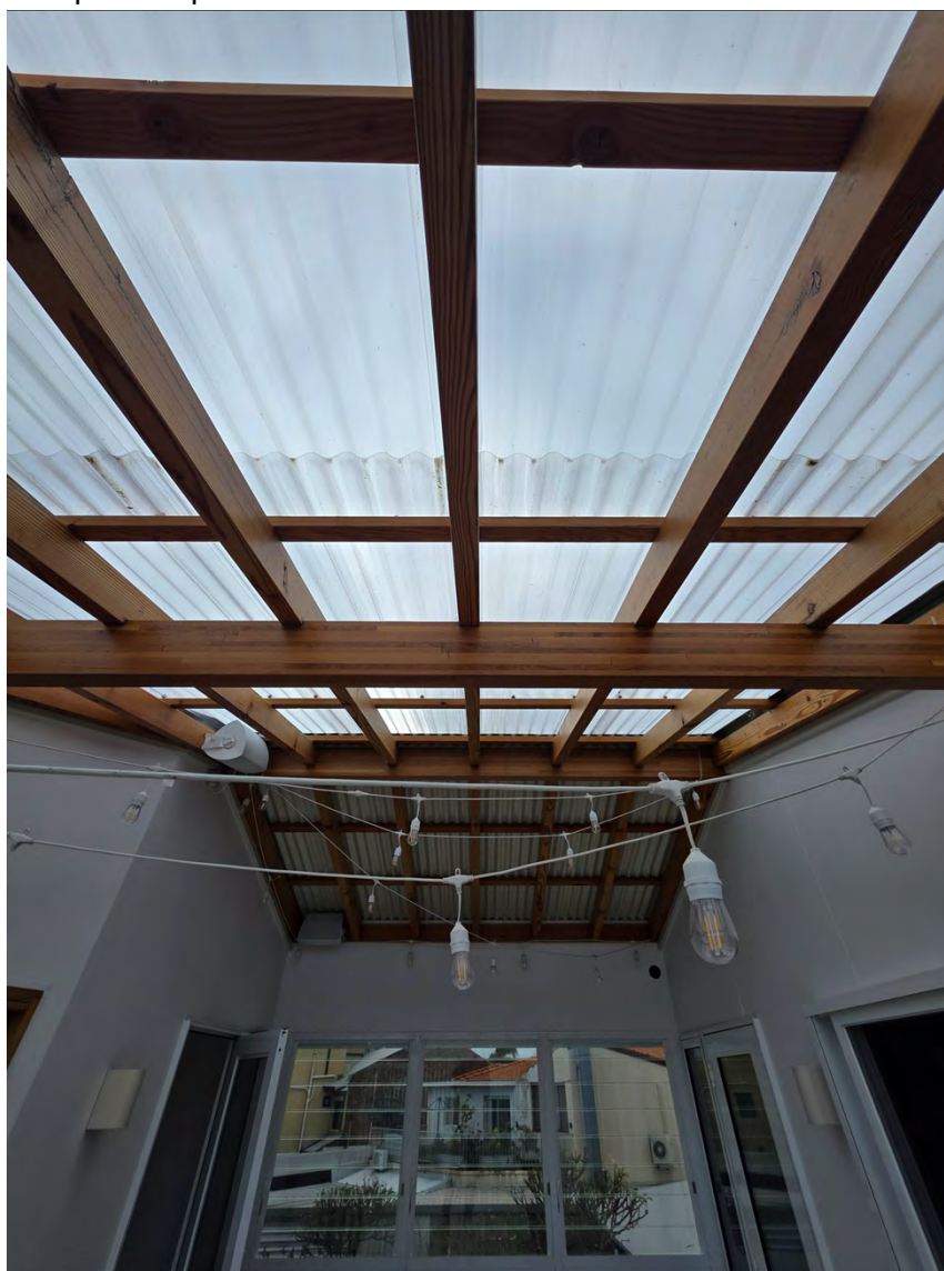
Image 1. Unauthorised roof sheeting additions (solid Colorbond sheeting to the northern face of roof and 'Laserlite 2000 (clear)' polycarbonate panel sheeting on the southern roof slope) to the first-floor terrace pergola. Image taken 1 July 2026.
